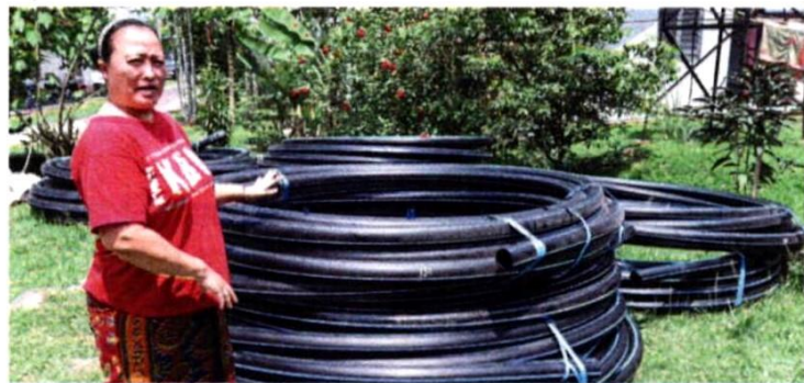
Hanim showing the pipes that are being installed in the village by Air Selangor to supply water to the homes.
